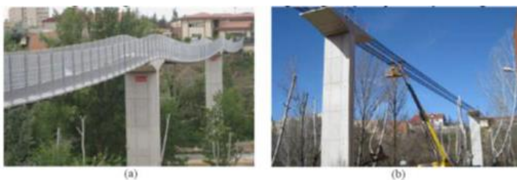
(a) View of the Cuenca footbridge; (b) View of the footbridge just after the FRP cable launching
